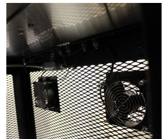
Vessel Cooling Fans
